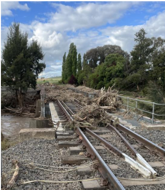
Plate B5.19 – (time unknown) Debris build-up on Molong Creek Railway Bridge.
