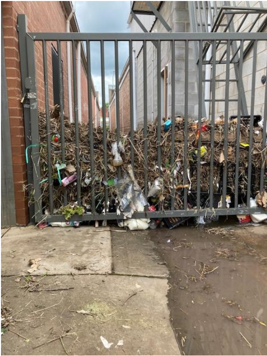
Plate B5.15 – (Photo taken at 14:30 hours) Debris build-up on gate between Molong Post Office and Supermarket.
